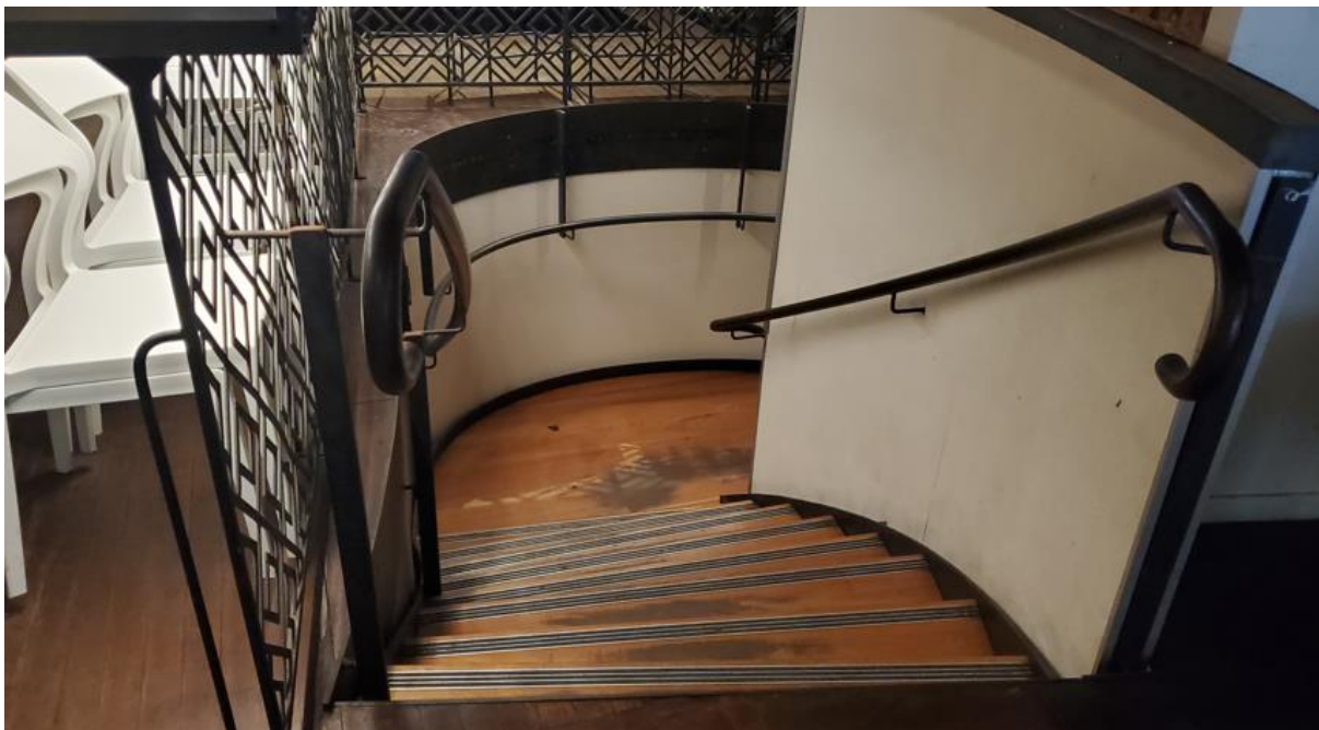
Figure 9: Existing stairs to basement level viewed from ground floor (proposed to be demolished as part of the subject application)
